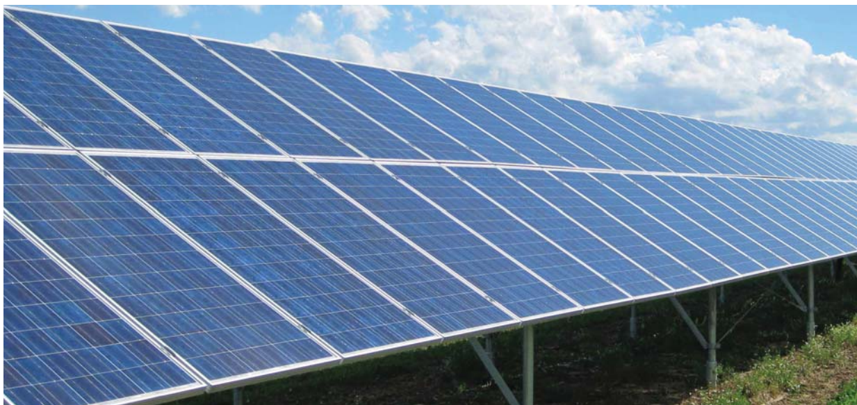
Ground Mounted PV
