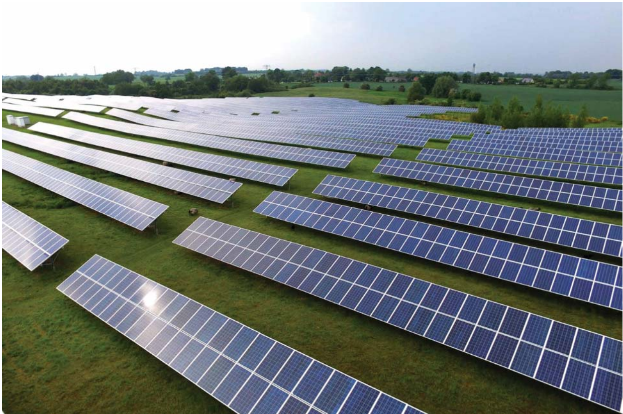
Typical solar farm
