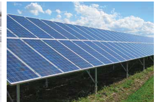
Ground Mounted PV
